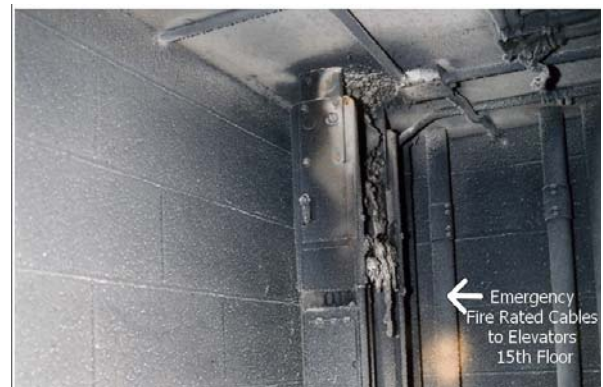
Figures 2: Fire rated cable installed in 3 inch conduit next to buss duct. (Note distance of conduit from buss duct)
